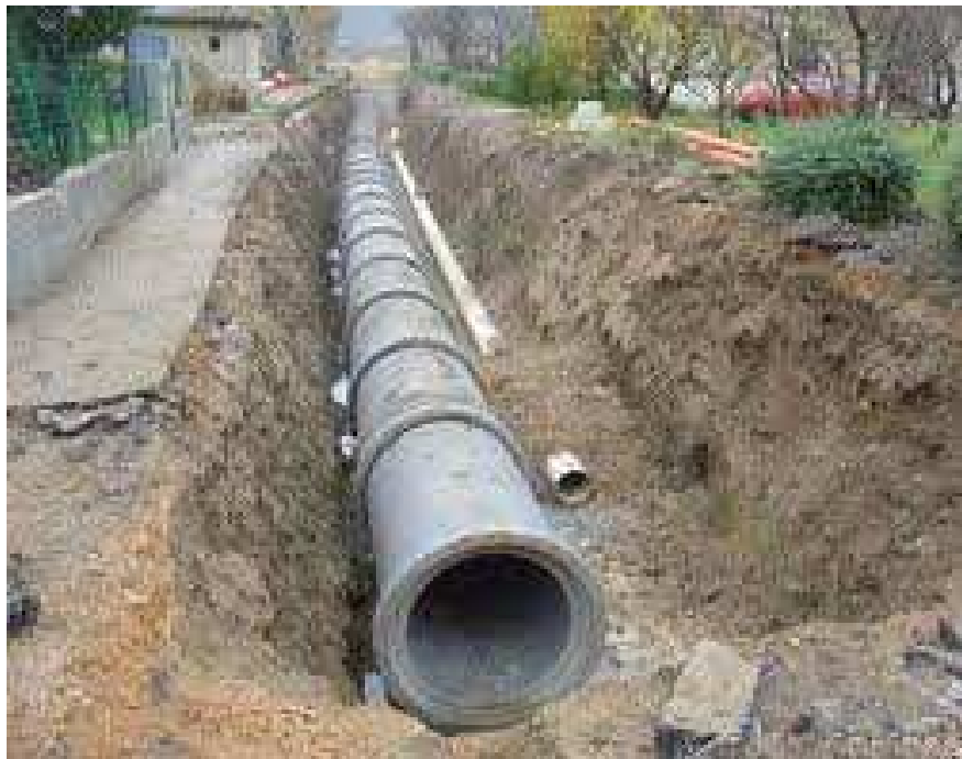
Concrete Sewerage network pipeline
