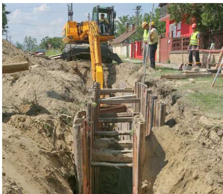
Escalation sewerage network pipeline in the street with wood suburb ,P.Bojovic Str.
