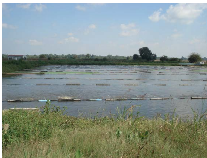
Bio lagune as wastewater treatment plant in the municipality of Velika Plana
