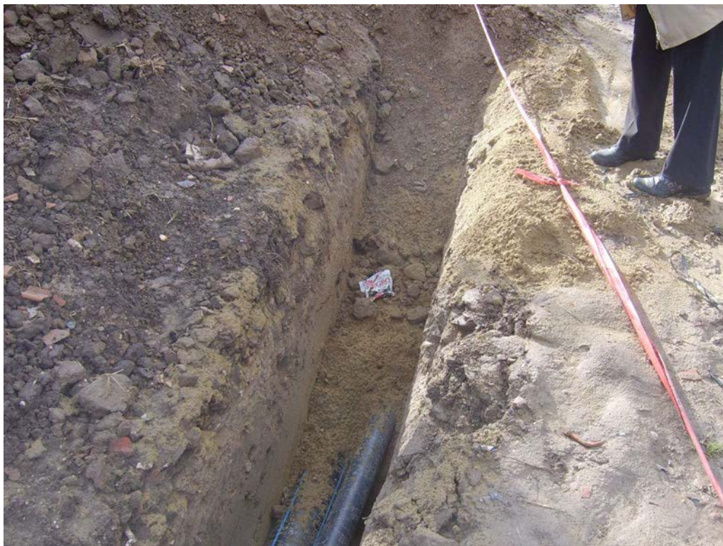
Water supply pipeline in Special Hospital For Mental Disorders "Dr. Laza Lazarevic", facilities in Padinska Skela
