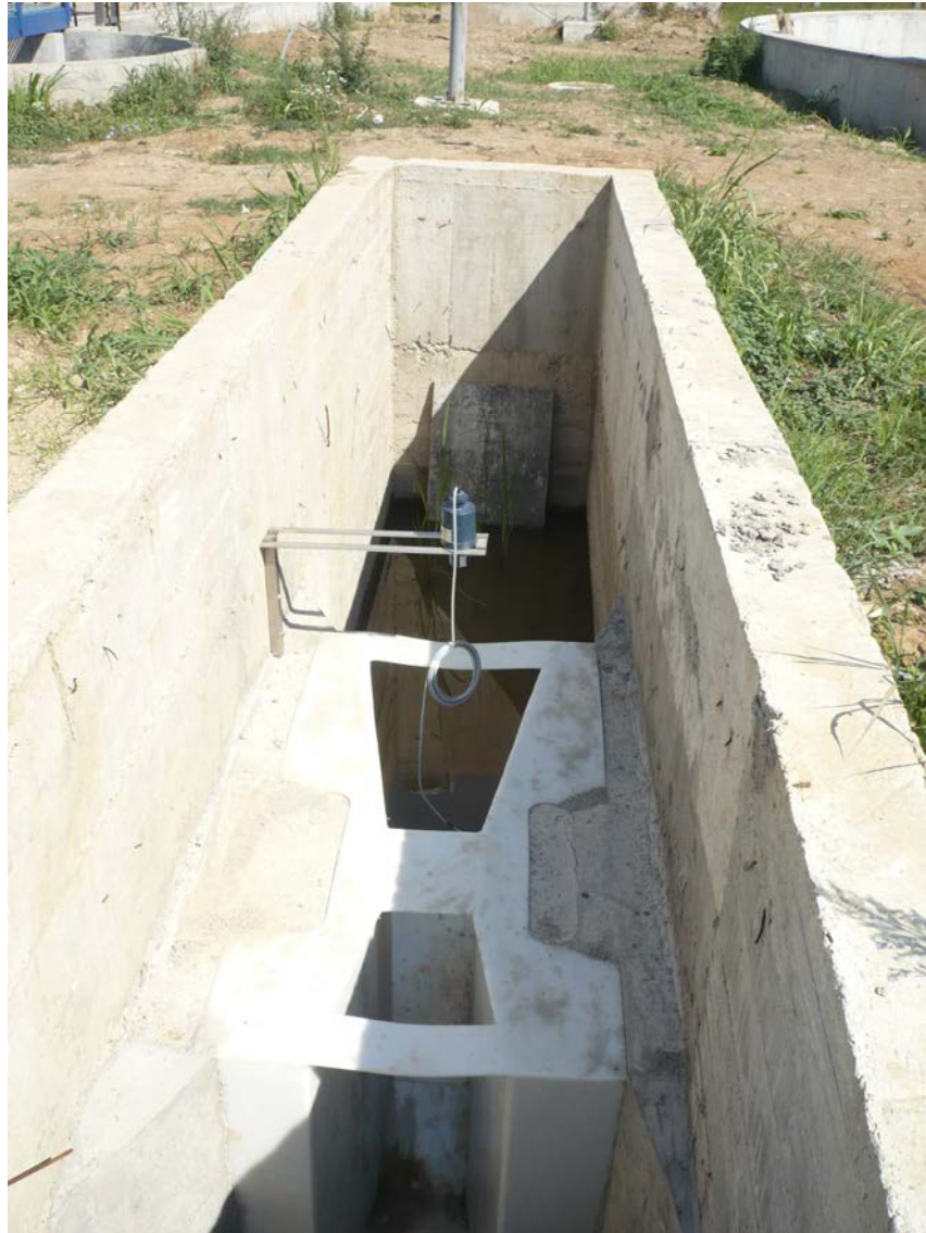
Waste water treatment plant Object of Flow meter
