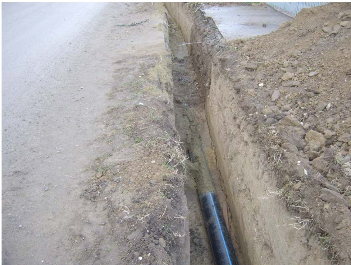
Water supply pipeline in Padinska Skela
